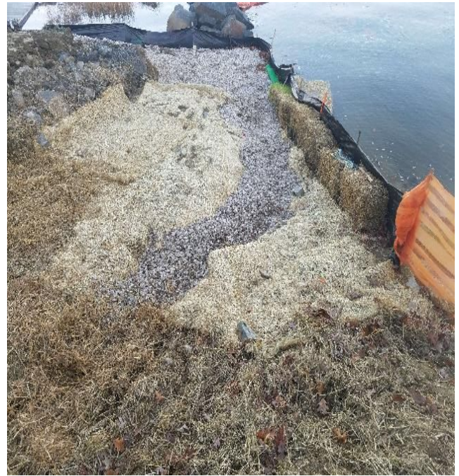
Fig 6: Stone swale installed next to trench at Getchell property/ West side of the Bay to divert water flow. Viewing east. (11-01-19).
