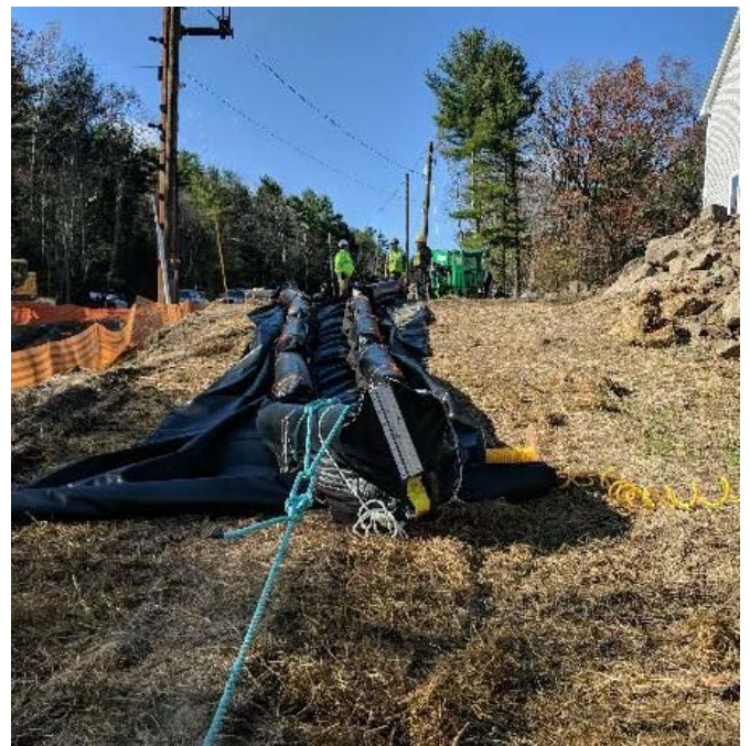
Fig 24: Turbidity barrier for hand jetting prior to installation at Getchell property - west side of the bay . Viewing west. (11-06-19).
