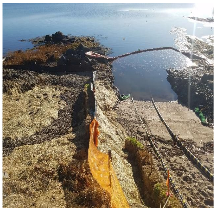
Fig 12: Two cables in trench at Getchell property/west side of the Bay. Viewing east. (11-02-19).
