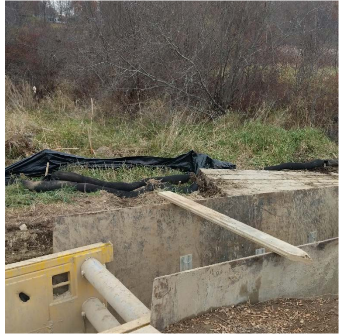
Fig 26: Silt socks replaced in kind at the Frink Farm at NW18. Viewing north. (11-06-19)
