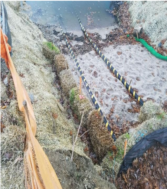
Fig 7: Bank stabilization in trench at Getchell property/west side of The Bay. Viewing east. (11-01-19).
