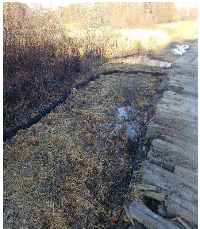
Fig 8: Filter sock installed around restored trench in NW 16 to protect Knights Brook tributary from sediment laden water. Viewing west. (11-01-19).
