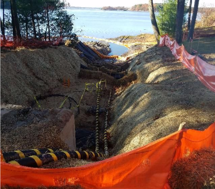
Fig 13: Two cables in trench at Gundalow landing/east side of the Bay. Viewing west. (11-02-19).
