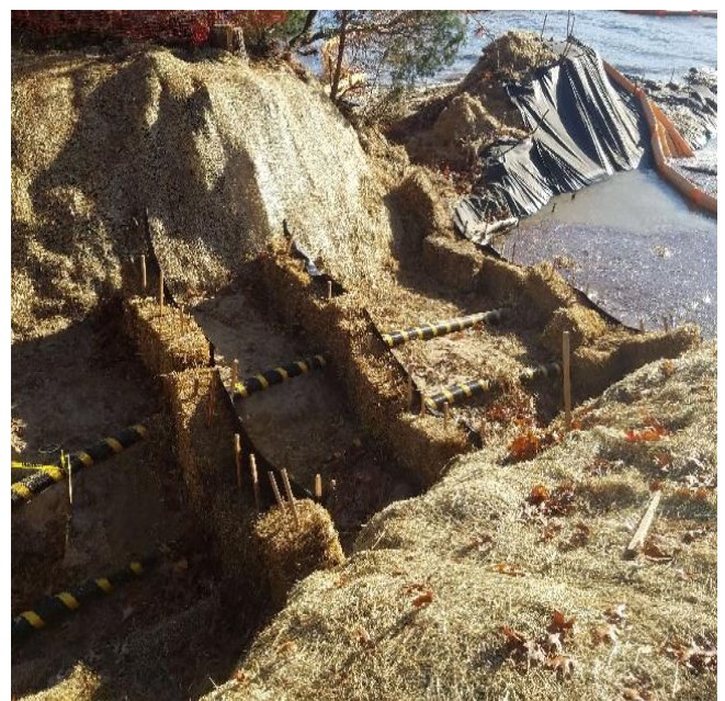
Fig 4: Triple row of sediment controls in trench at Gundalow Landing/ east side of the Bay. Viewing west. (11-01-19).
