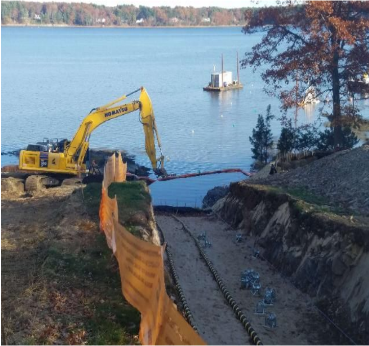
Fig 17: Floating cable across the Bay. Viewing east. (11-04-19).
