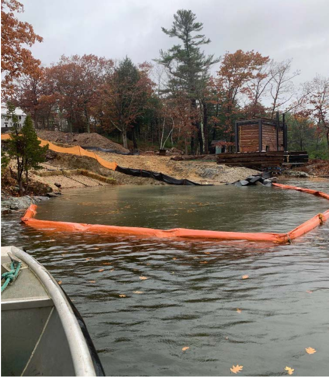
Fig 1: Silt curtain repaired on the Getchell property/west side of the Bay. Viewing west. (10-31-19).
