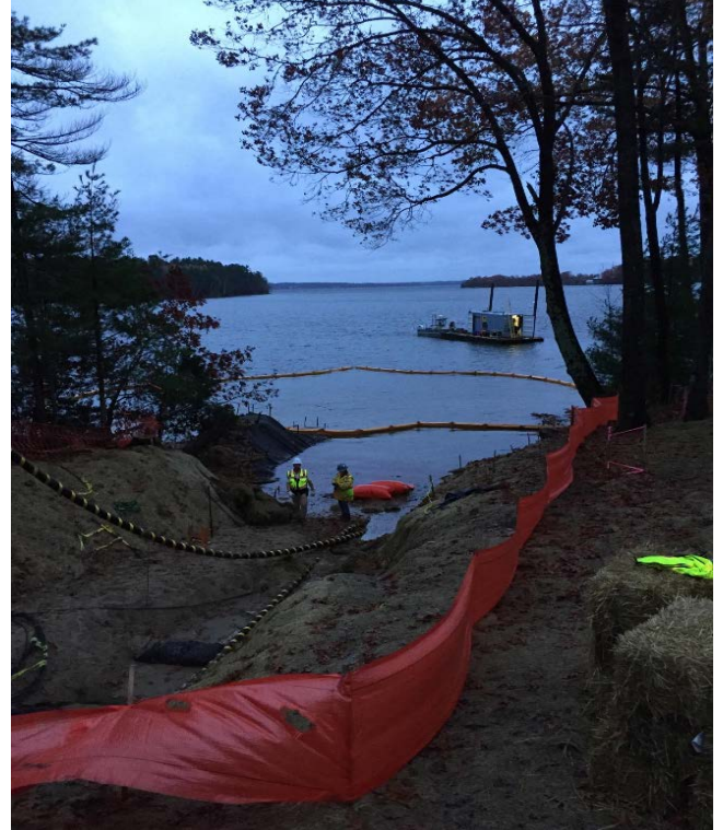
Fig 2: Silt curtain re-installed at Gundalow landing/east side of the Bay after pulling in Cable 2. Viewing west. (10-31-19).
